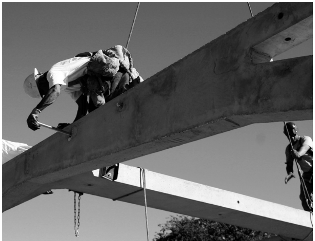
Erection crew workers with Jett Enterprises bolt together steel rods that tie the concrete frames into place.
